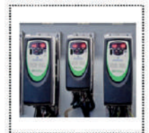
Automatic inverters Brand: Emerson in USA
